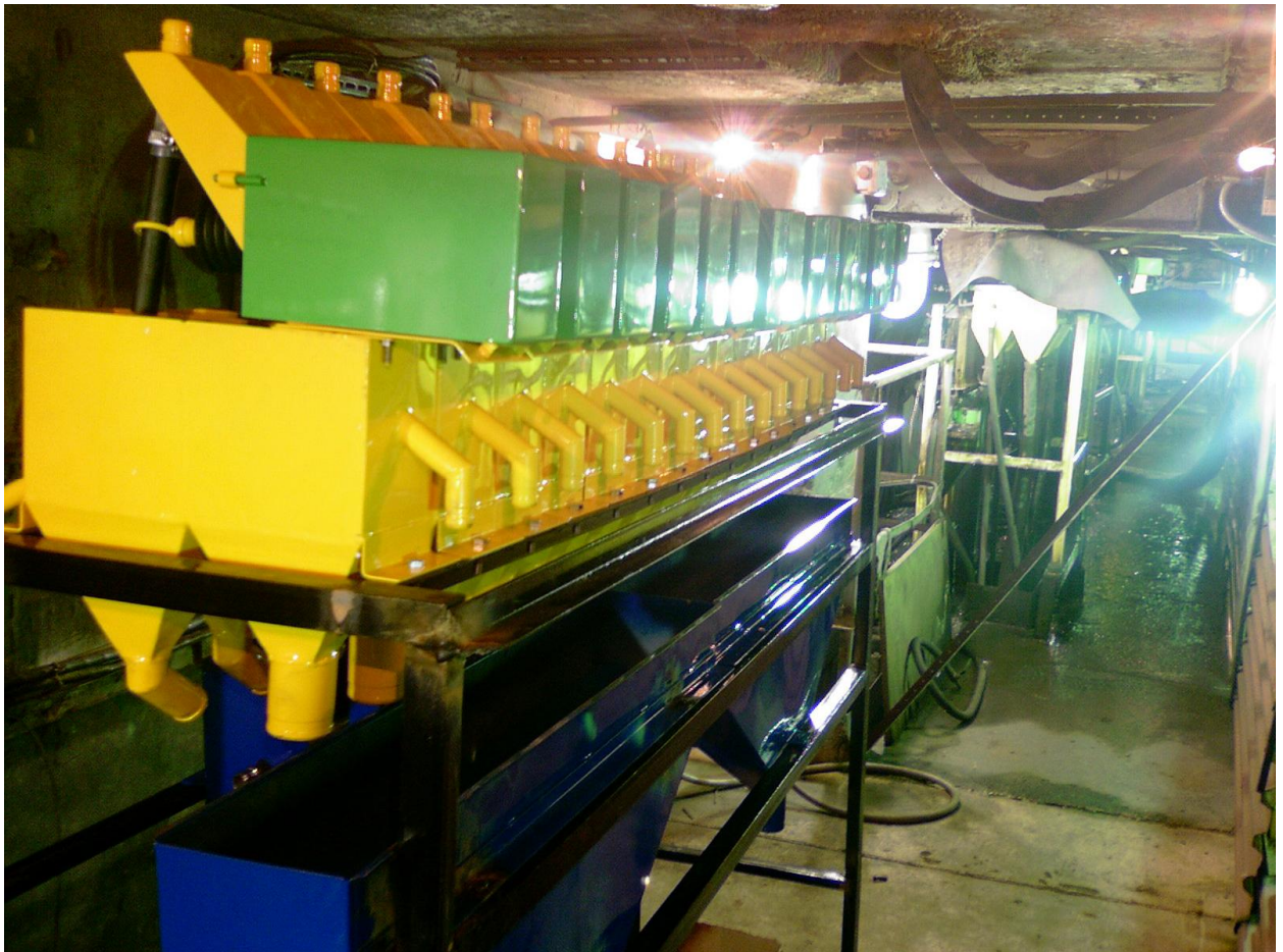
The photo of the multiplexing station (for the “Courier-6” XRF analyzer) designed and made by Uralautomatica Engineering specially for Norilskiy Nickel
